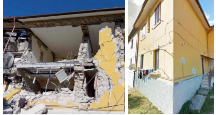
Pre- and post-earthquake damage to a building. Photo: Massimiliano Stucchi
