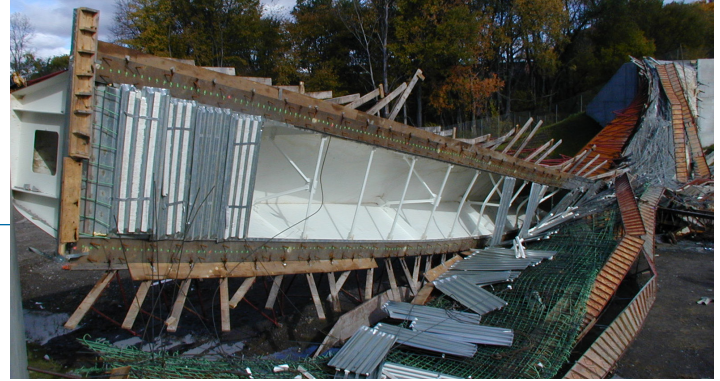
Failure of box girder during construction. Photo: Robert Ratay
